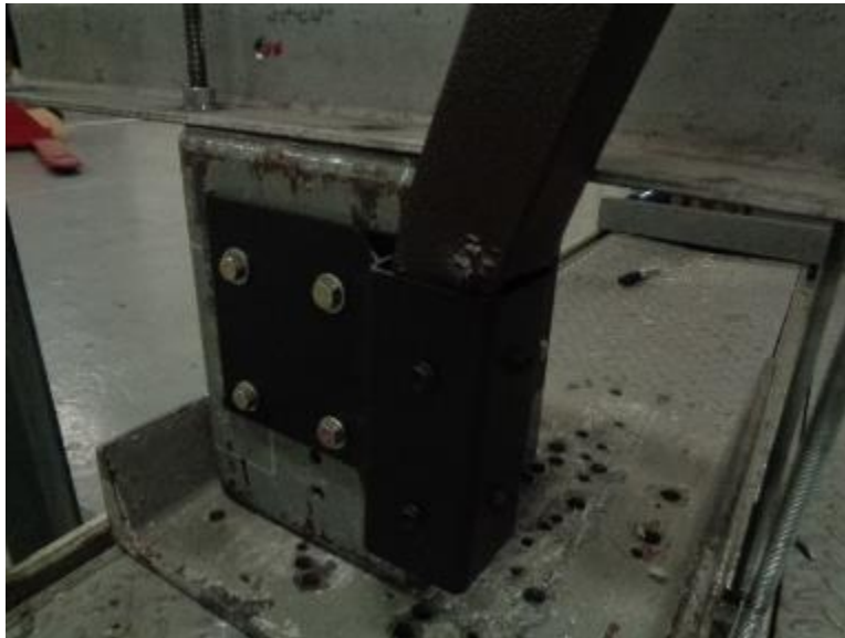
Photo No. 3 Typical Failure - Buckling of Post above Bracket
