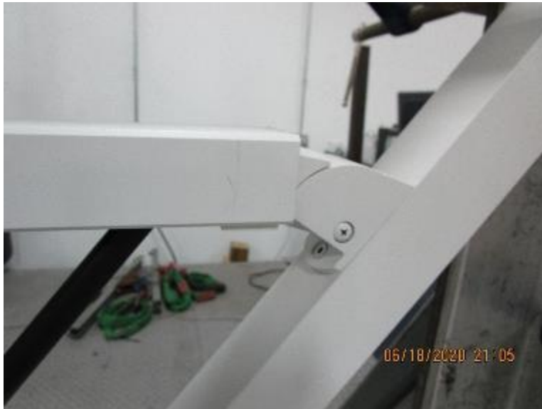
Photo No. 10 Stair Rail Bracket
