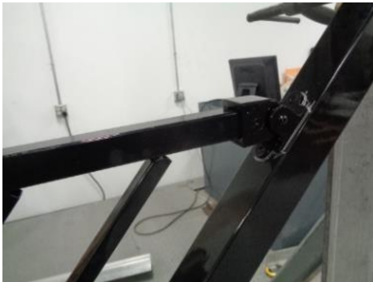
Photo No. 6 Stair Bracket Attached to Fe26 Post
